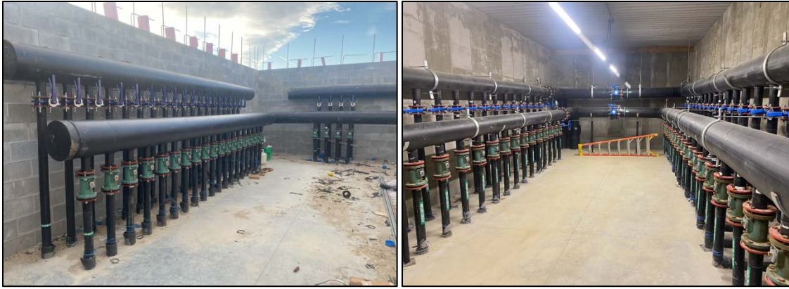
Figure 11a (left) & 11b (right): Examples of distribution manifolds with shut-off valves and balancing valves installed within mechanical rooms
