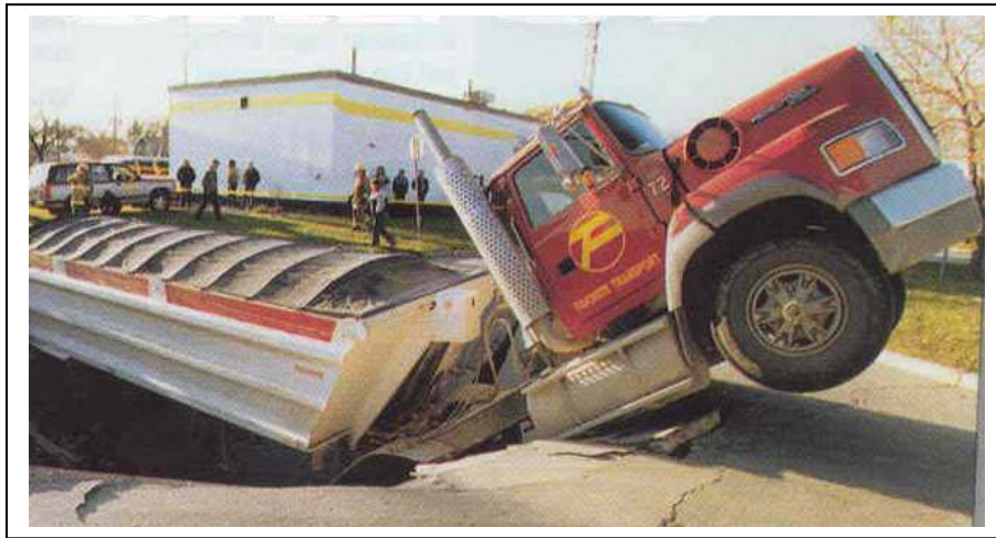
Sinkhole from Joint Infiltration
