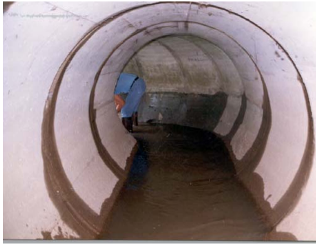
Concrete Pipe Joint Leaks Every 8-feet
