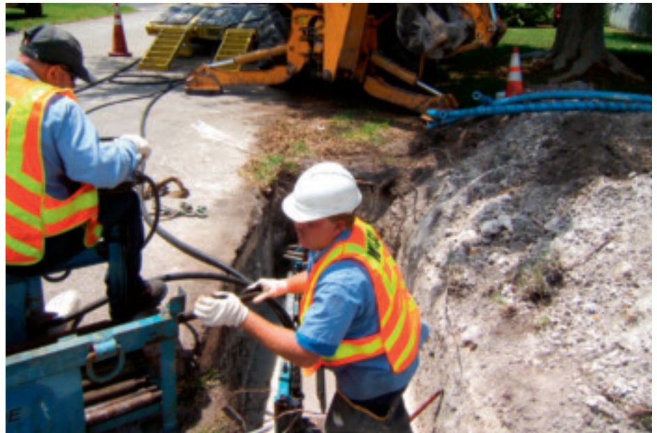
Miami-Dade’s two-man crew easily installs a new 2-inch HDPE water pipe-line. In just a few hours, residents have water pressure returned to normal.
