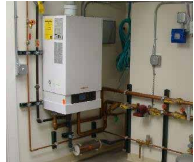
This system will use a dedicated boiler
