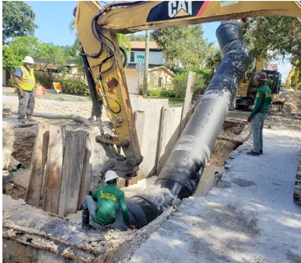
Contractors moved at unparalleled speed to build an entire new line, completing the job months ahead of schedule
