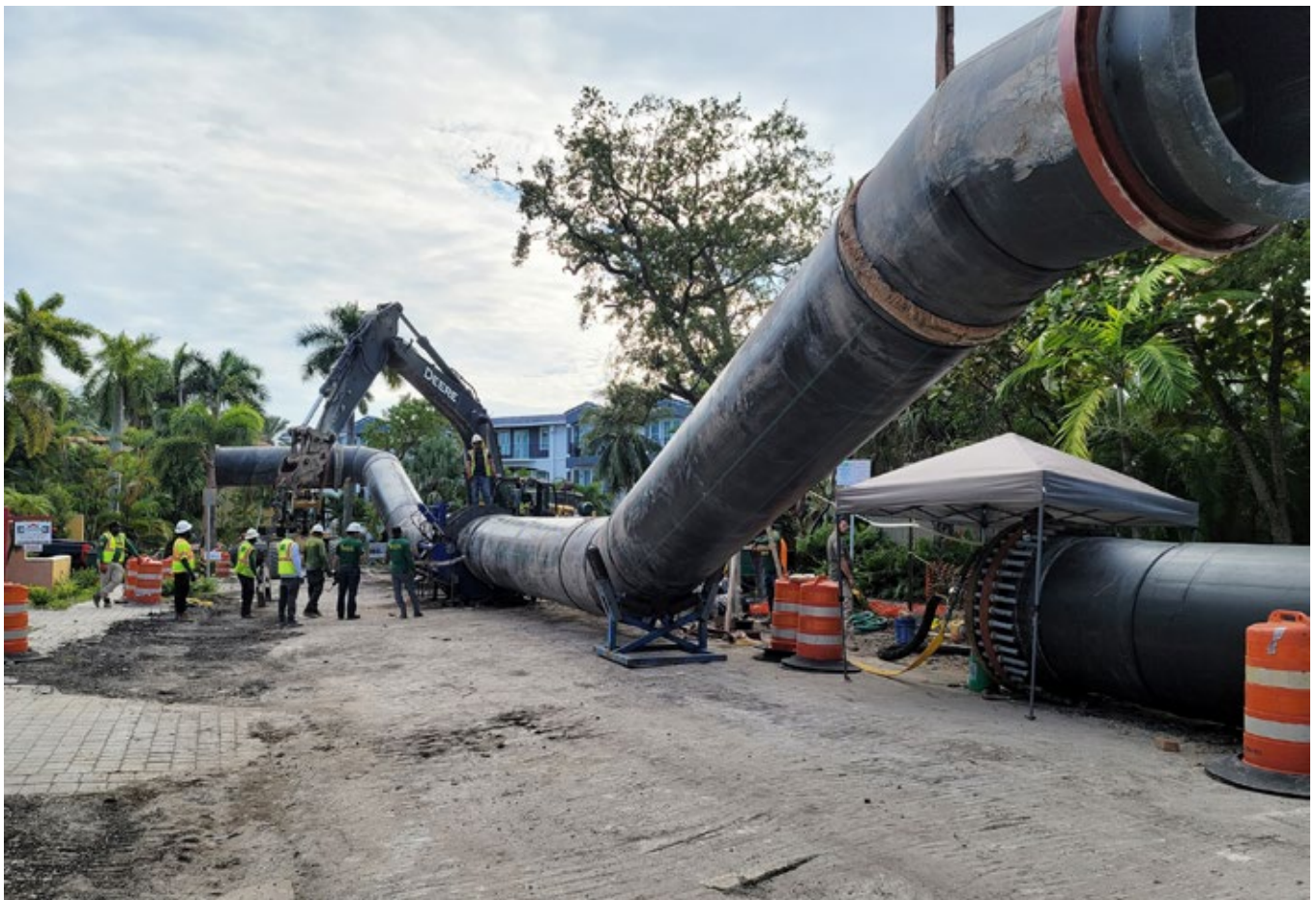
Four of the HDD segments required unique compound curves due to roadway geometry and field conditions
