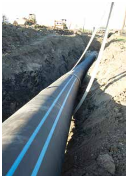
Hydrotesting can be used on runs of HDPE pipe that are hundreds of feet long
