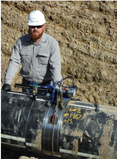
The new PPI TN-60 report discusses non-destructive testing methods such as this field inspection of the fused joint of two sections of 24-inch diameter DR9 PE 4710 pipe using the Evisive MW Band Scanner. Photo courtesy of Evisive.
