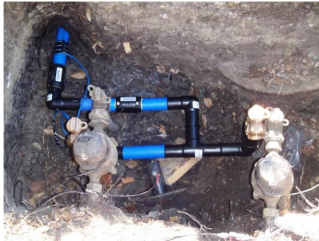
Fig.3: Fused Meter Manifold with Transition to Brass at Meter Inlet
