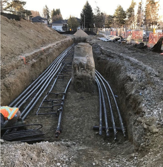
Parallel HDPE pipes installed as part of a buried geothermal header system. Photo courtesy of Geosource Energy Inc.
