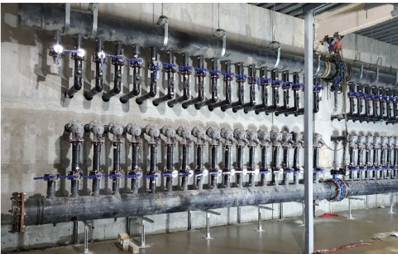
The construction of large HDPE manifolds for a commercial geothermal system. The new PPI MS-7 provides detailed language for specifying both outdoor and indoor GSHP piping systems. Photo courtesy of Geosource Energy Inc.
