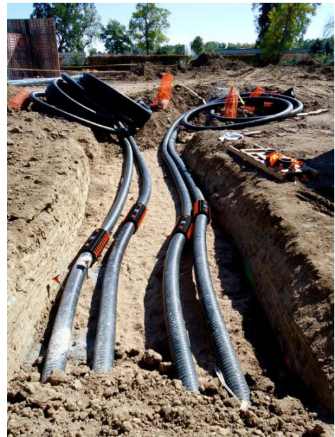
Four parallel, five-inch diameter, pre-insulated PEX pipes are laid out side-by-side for supply of heated fluid for snow melting and radiant heating within the new Asian Tropics complex. These flexible pipes follow the contours of the land over long distances.
