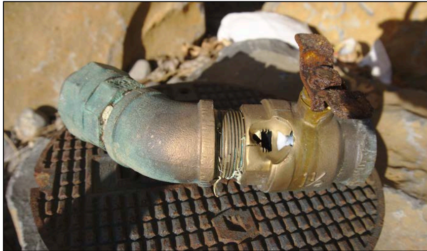
Figure 6: Brass water valve that is partially melted
